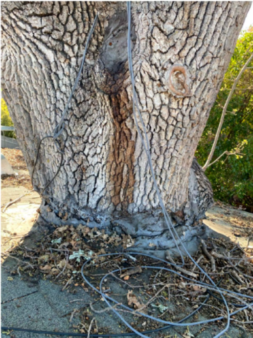
Photo 3. Tree #75 emerging from the roof of Unit 111.
