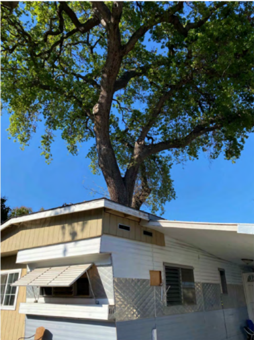
Photo 2. Tree #75 grows through the floor and roof of Unit 111.
