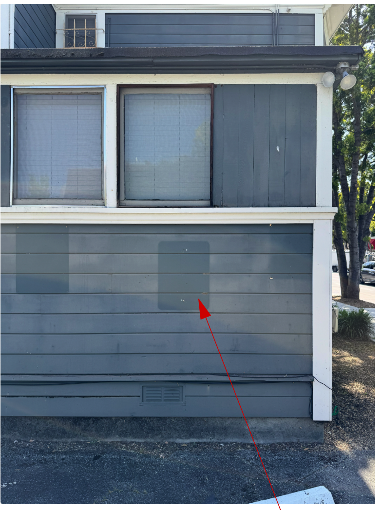
7 REHABILITATE SIDING WHERE SIGNAGE REMOVED AND DISCOLORATION IS PRESENT
