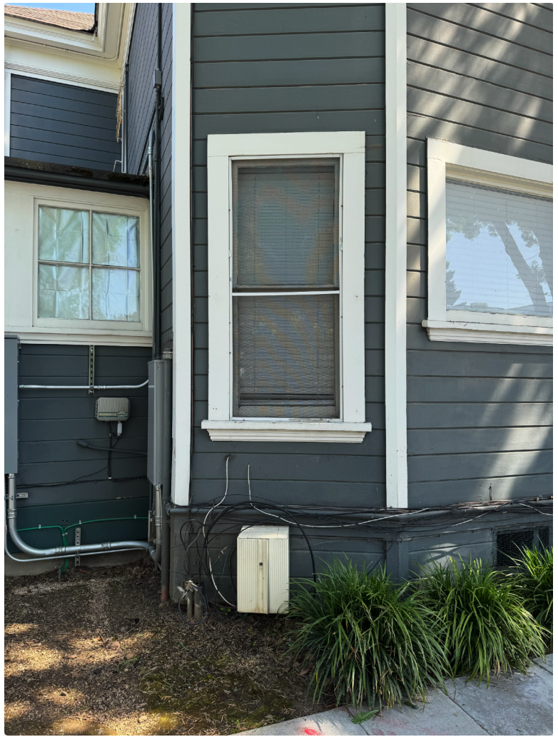
15 INVESTIGATE CABLING /WIRES AND SECURE IF STILL IN USE, TYP.
