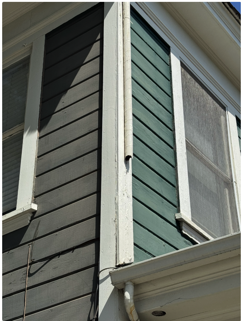
3 INVESTIGATE DOWNSPOUT CONNECTION TO EXISTING UPPER ROOF GUTTER AND ASSES FOR REHABILITATION
