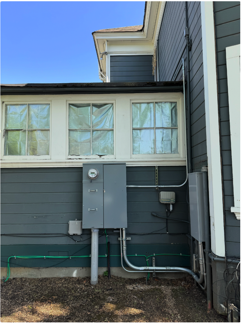
9 INVESTIGATE CONDUIT /CABLING /WIRES AND REMOVE IF NOT IN USE, TYP.
