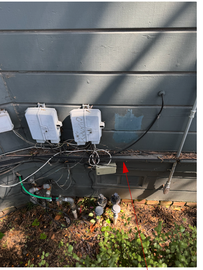
11 INVESTIGATE CABLING /WIRES AND SECURE IF STILL IN USE, TYP.
