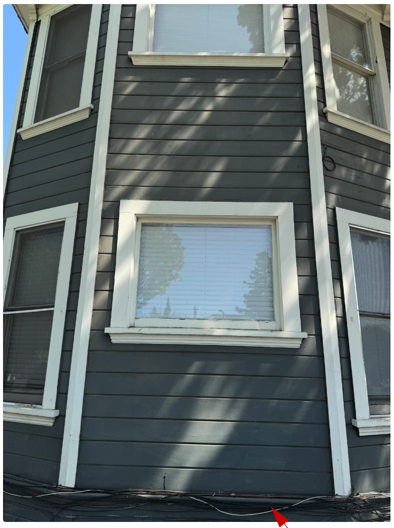
13 INVESTIGATE CABLING /WIRES AND SECURE IF STILL IN USE, TYP.
