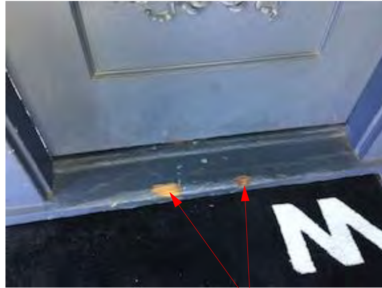
5 REPAIR CHIPS IN WOOD DOOR SILL
