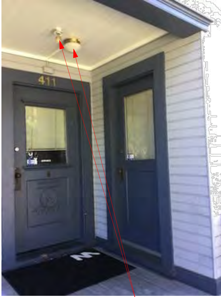
3A REMOVE LARGER UNORIGINAL LIGHT FIXTURE & REPLACE GLOBE OF SMALLER ORIGINAL LIGHT FIXTURE
